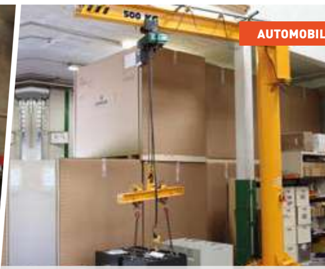
Potence et palan – Manutention de batteries
